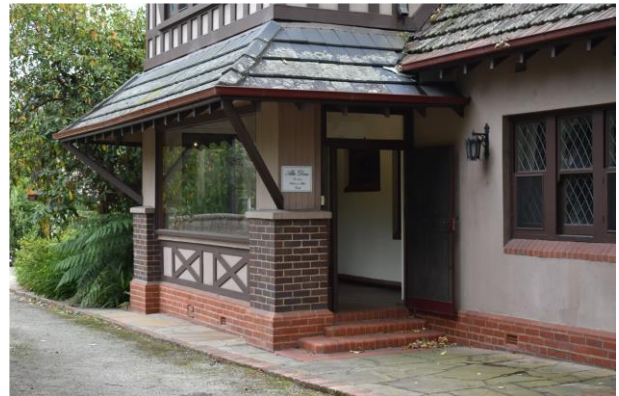
Detail view of entrance portico and awning (source: Extent Heritage Pty Ltd, 2022).
